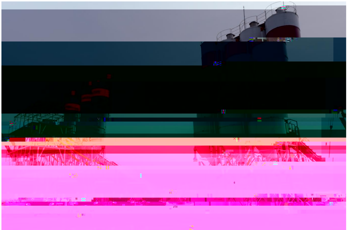
CAPTION: The Megawide mobile concrete batching plant in Apalit, Pampanga, built to supply concrete for the Malolos-Clark Railway Project Package 1
